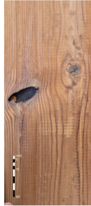
Knotholes A grade: Not allowed B grade: Allowed, up to Ø 20 mm, max 1 pc. x board length, m
