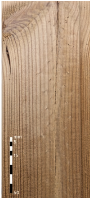
End splits A grade: Allowed, up to board width B grade: Allowed, up to 300 mm
